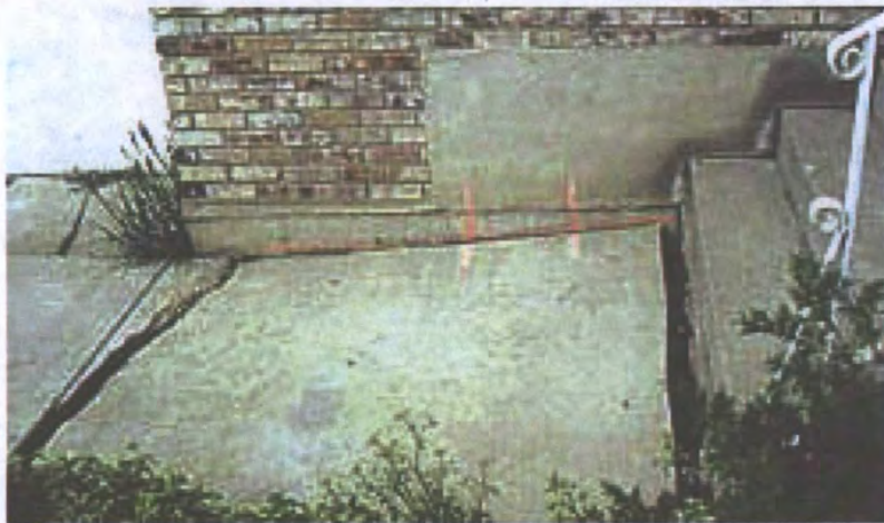
Figure 37. Sidewalk pulling away from house. (Photograph courtesy of Utah Geological Survey.)
