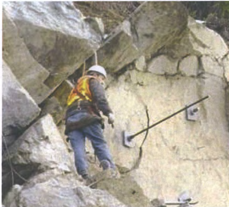
Figure C33. A rock bolting operation; notice broken-up (crumbling) nature of the rock. (Photograph by Washington Department of Transportation, USA.)
