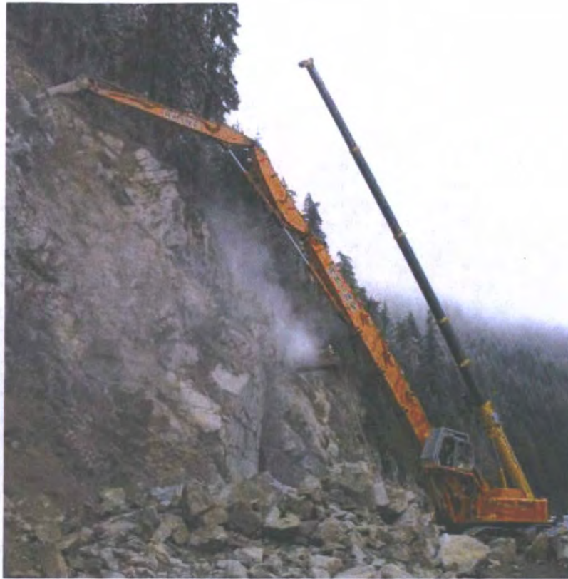
Figure C30. A hydraulic rock hammer in action, bringing down rock from the slope. This is an alternative to blasting rocks down. (Photograph by Washington Department of Transportation, USA.)
