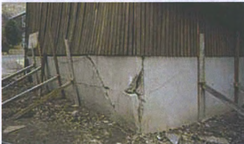
Figure 38. Cracking of the foundation of a structure. (Photograph courtesy of Utah Geological Survey.)
