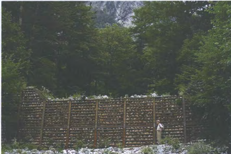
Figure C37. A debris-flow retaining wall in Kamikochi Basin, Japan. (Photograph courtesy of Goncalo Vieira.)
