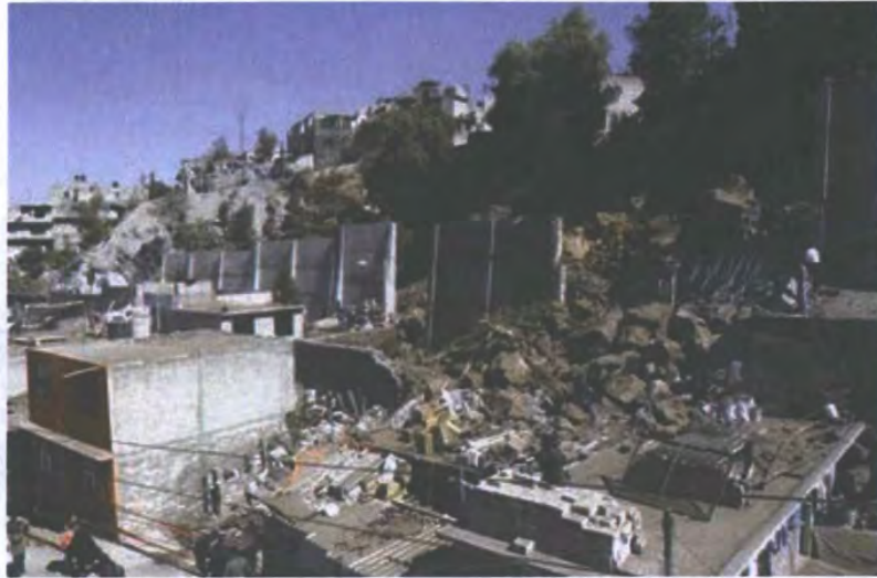
Figure C36. Caution is required in locating and constructing debris-flow retaining walls. This is a photograph of the partial failure of a retaining wall, caused by a landslide in Iztapalapa, a suburb of Mexico City, Mexico. The landslide slid onto a house at the toe of the slope, killing two people, and was triggered by heavy rains in the area. The house was below the 5-meter-high (15 yards) wall, but the wall could not withstand the mass of rocks and soil. (Photograph by Chinagate/Xinhua.)
