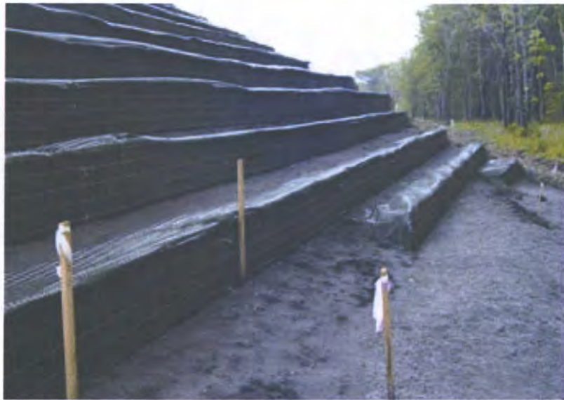
Figure C4. Schematic and photograph of a lightweight backfill. There has been an increased growth in the use of recycled tire shreds in civil engineering applications. Highway applications include using shredded tires as lightweight fill over weak soils in bridge embankments and retaining wall reinforcements or, in very cold climates, as insulation of the road base to resist frost heaves and as a high-permeability medium for edge drains. (Graphic from reference 11, photograph from U.S. Department of Transportation, Federal Highway Administration.)
