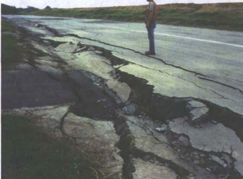
Figure 12. Photograph of lateral spread damage to a roadway as a result of the 1989 Loma Prieta, California, USA, earthquake. (Photograph by Steve Ellen, U.S. Geological Survey.)
