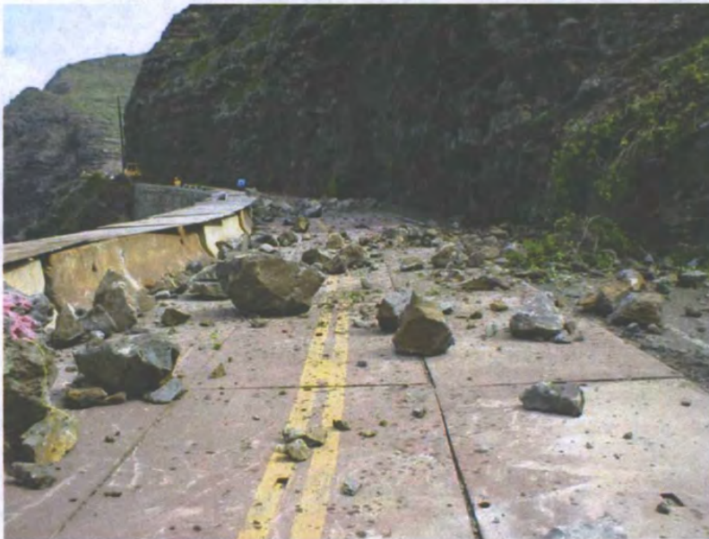
Figure C29. Rocks dislodged by scaling and blasting. (Photograph by Washington Department of Transportation, USA.)
