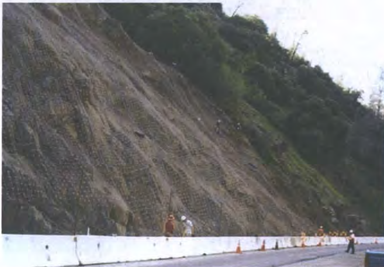
Figure C21. Example of wire mesh placed over a rocky slope to contain the rocks that may come down.
