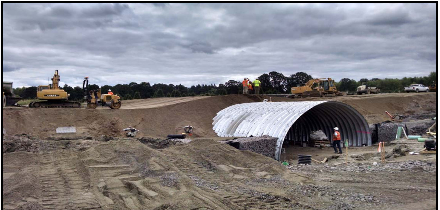
NE 119th Street (NE 72nd Avenue to NE 87th Avenue), including a new Curtin Creek Culvert
